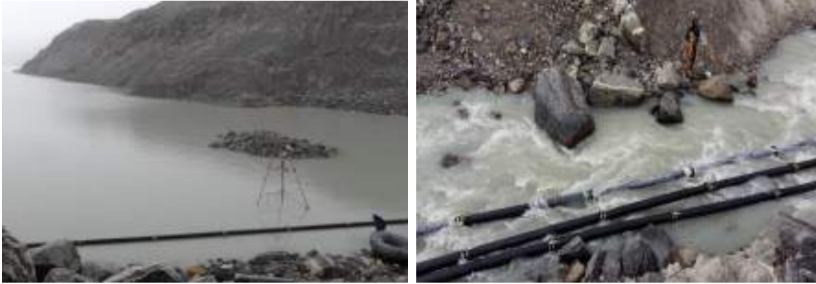
I. GLOF sensor installed in South Lhonak Lake & II. Pipelines laid down for the siphoning of water from South Lhonak Lake
