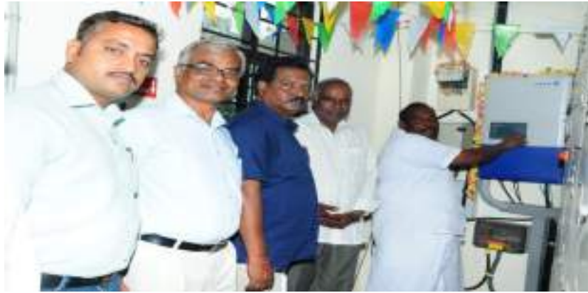
5.13. A view of the power plant installed at the terrace of Dr. Abdul Kalam Science Centre
