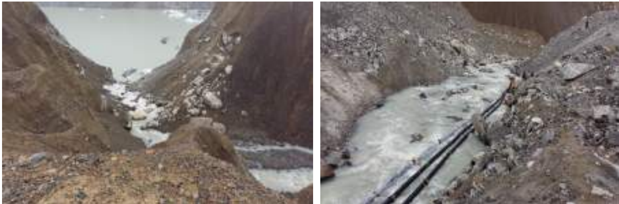
I. Photograph showing the stream draining to the South Lhonak lake & II. The photograph showing laying of pipelines with the help of rope in September 2016
