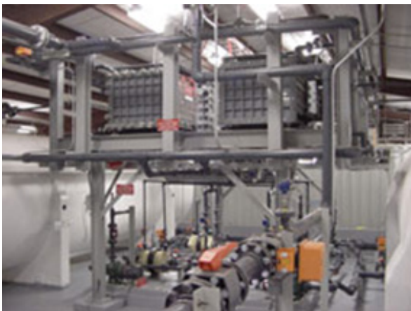
(170 kW/1 MWh unit, Sumitomo electric industries in Japan; Open Source)
