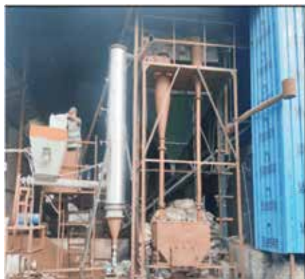
Fluidized bed gasifier at New Raj Food Industry, Dahod
