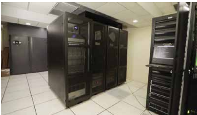
High Performance Computing facility
