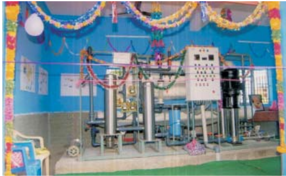
Fig. 4.37: Water Purification Unit at Thiruppattur (Tamilnadu)
