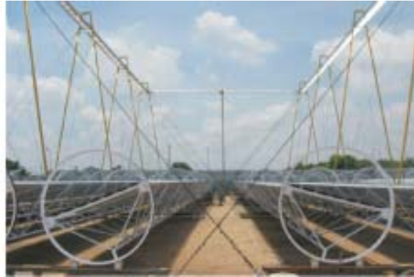
Fig. 4.40: Existing solar collector system in coimbatore
