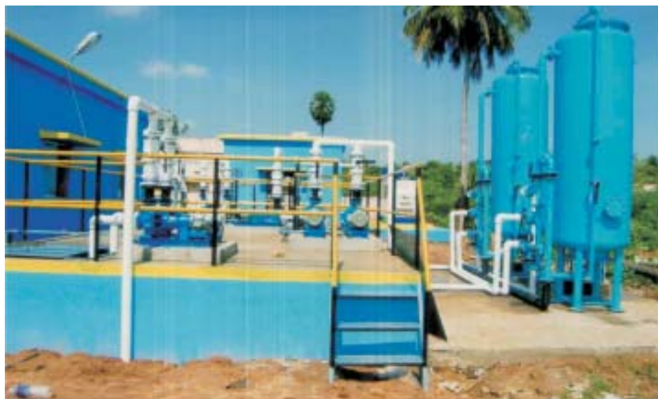
Fig. 4.36: Water Pre-treatment Unit at Mamsapuram (Tamilnadu)
