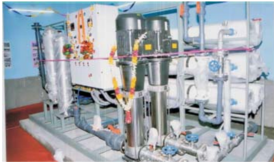
Fig. 4.35: Water Purification Unit at Mamsapuram (Tamilnadu):
