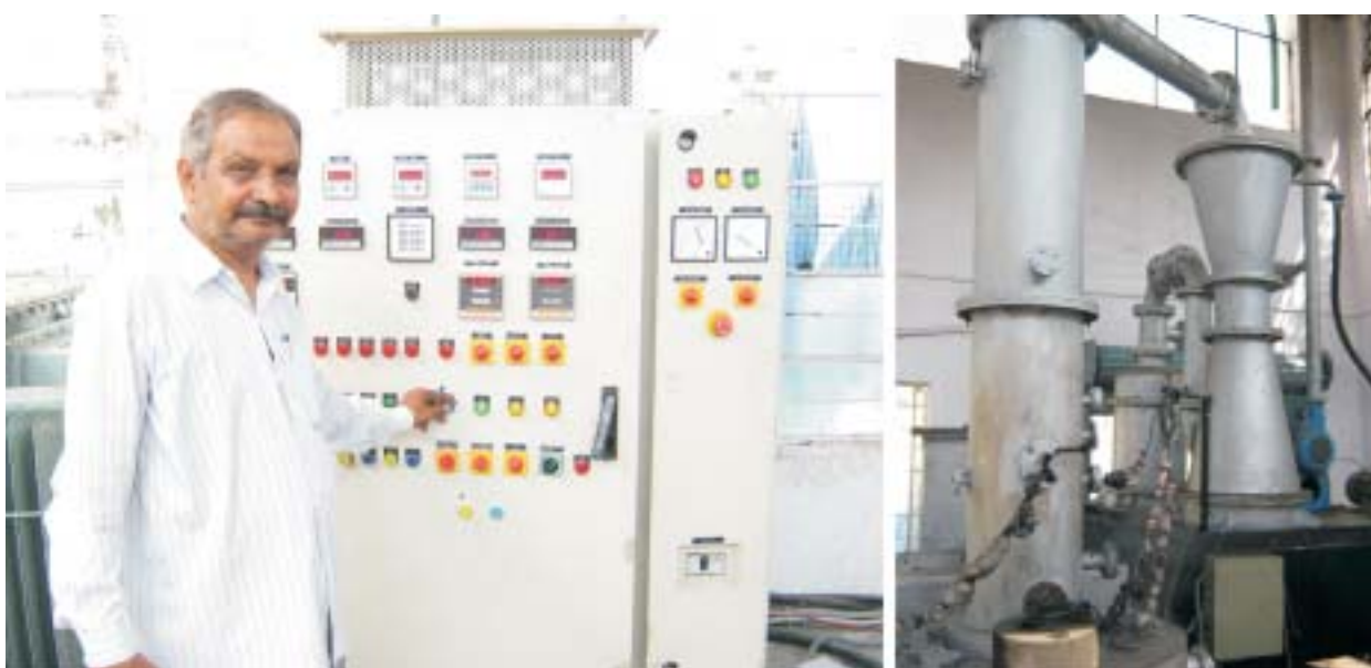
Fig. 4.43: Plasma Pyrolysis System (Green Technology) installed at GCRI, Ahmedabad
