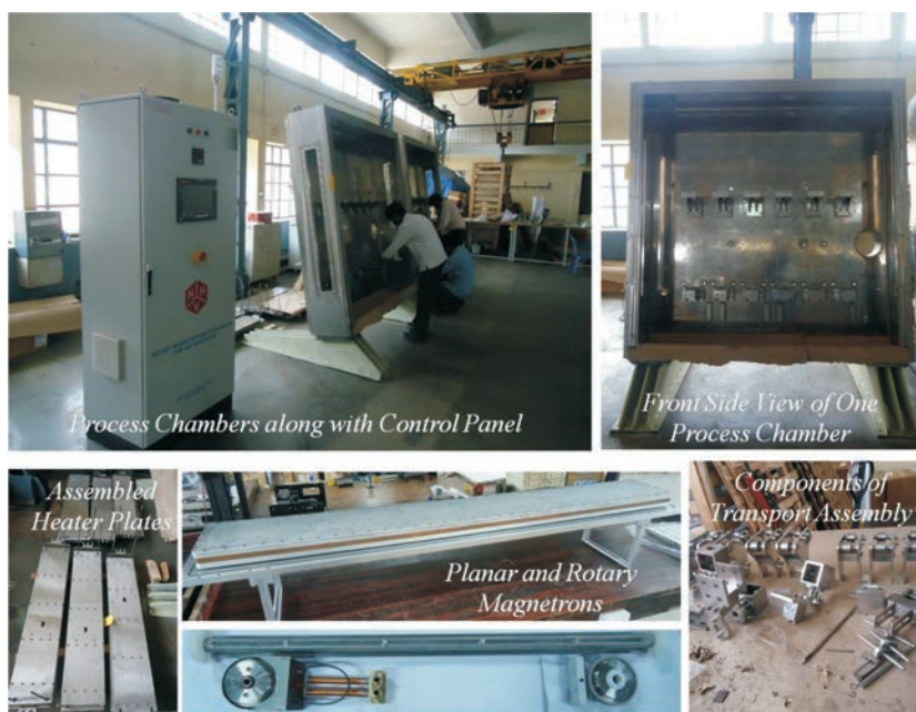
Assembly of Sputtering System for large area substrate
