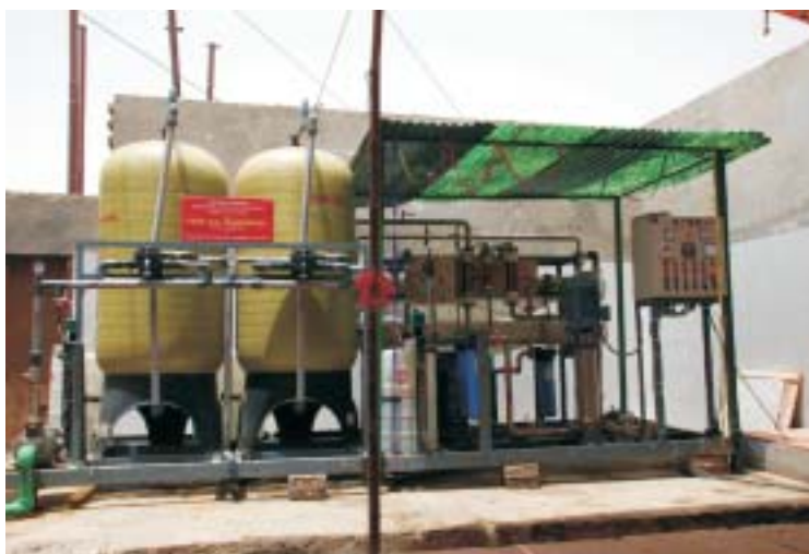
Low Energy Membrane Desalination & Defluoridation plant installed at HCST Campus, Farah , Mathura
