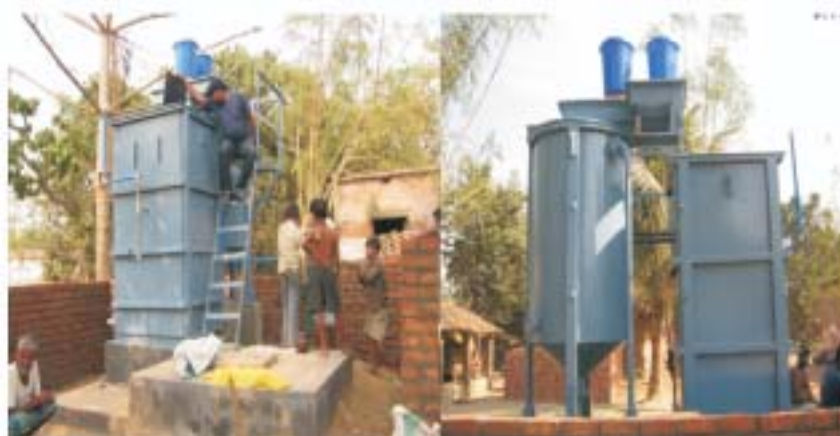
Community Based Arsenic Removal Plant at Maltipur
