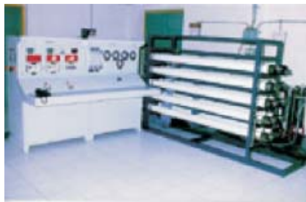
Two Stage Reverse Osmosis System
