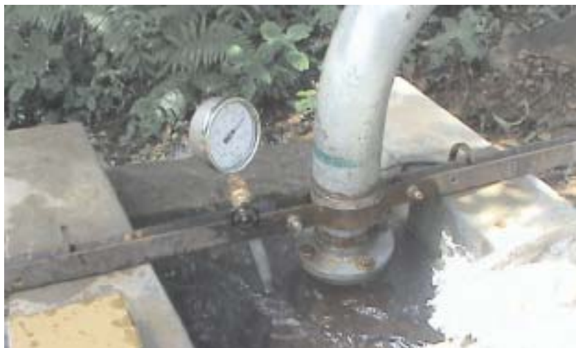
Fig. 1.9 : ‘Pump as Turbine’ – A project under implementation
