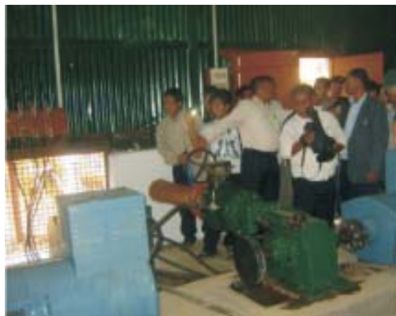
Fig. 8.2: Micro Hydel Power Plant in the Power House at Dailong Village, Manipur
