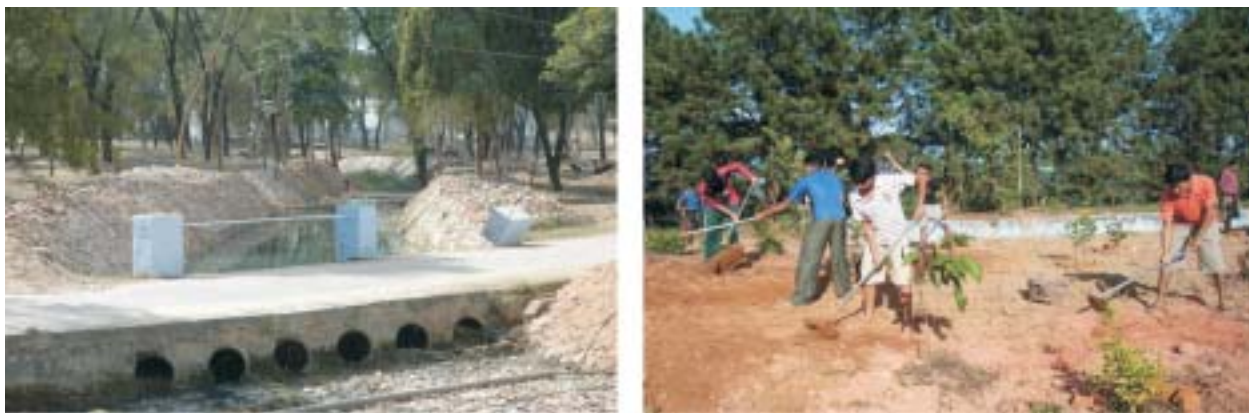
Fig. 5.2 : Local solution with local resources through a judicious combination of TK and S&T : School kids involved in land and check dam preparation
