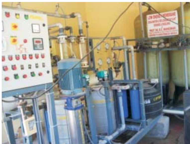
Fig. 8.3: Low Energy Membrane Desalination & Defluoridation Plant installed at Nagla Chandrabhan Village, Mathura, U.P.
